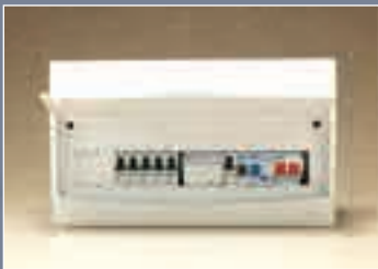
LHZ Control box
